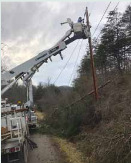
The crew utilizes a digger truck to secure a pole while conductors are being repaired and reattached to the pole. Photo: Roger Auxier
