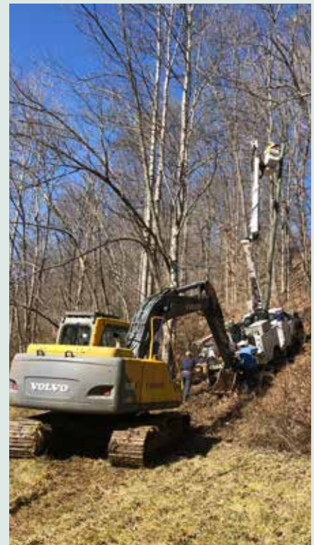
A track hoe assists crews in getting a bucket truck to a pole so they can repair conductors. Photo: Roger Auxier
